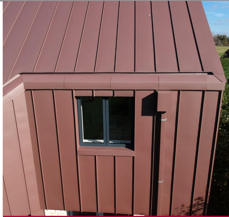
The eaves gutters are pulled back to create a shadow gap along the edge of the roof and free the eaves up from rainwater collection, contributing to the effect of the cladding running over the roof.
