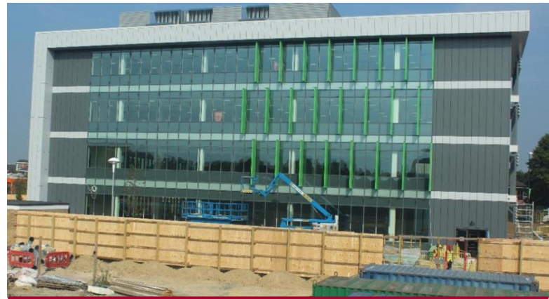
The AH-25 system was applied over a concrete substrate with a bituminous vapour control layer.
