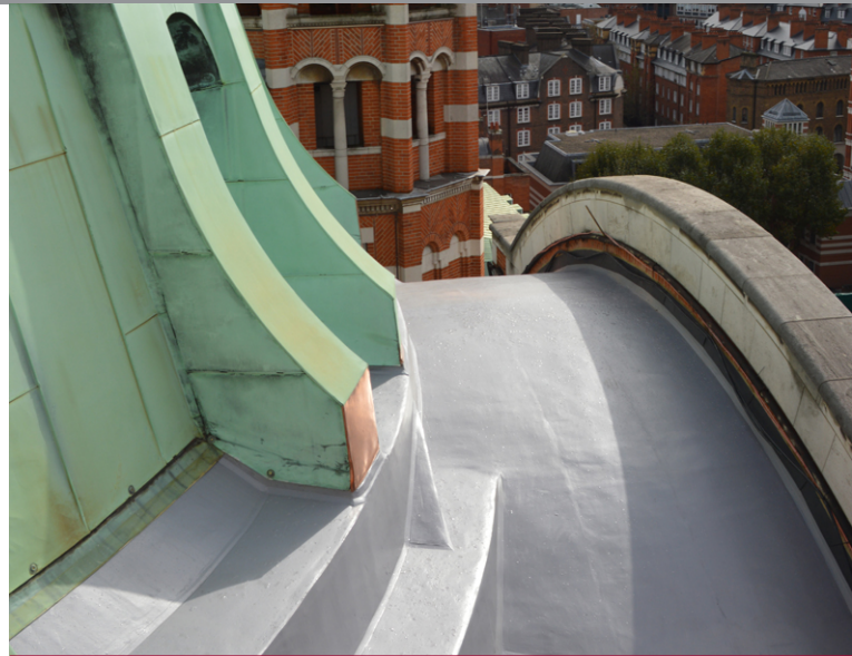
IKO's Permaphalt – a polymer modified mastic asphalt – was specified for the extensive reroofing of the Roman Catholic Cathedral.
