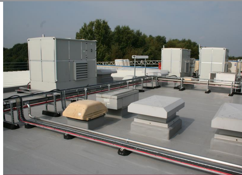
The refurbished roof of the Doncaster Vue – all the interfaces competently dealt with using AH-25
