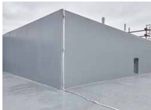
Top Visualisation of the completed school. Above Single ply was used to cover a storey-high change in roof height at Arnold Hill, removing the need for a render finish.
