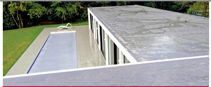
IKO Armourplan P PVC Single Ply Membrane flat roof application illustrating the clean uncluttered finish.
