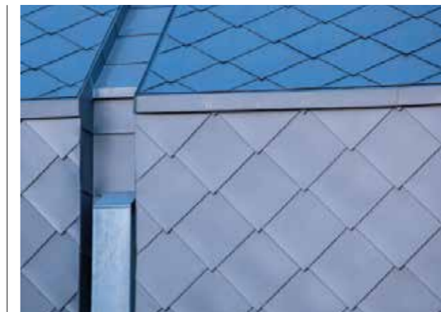
Opposite page The amphibious house with its distinctive NEDZink shingles looks anything but – until the nearby river floods.
