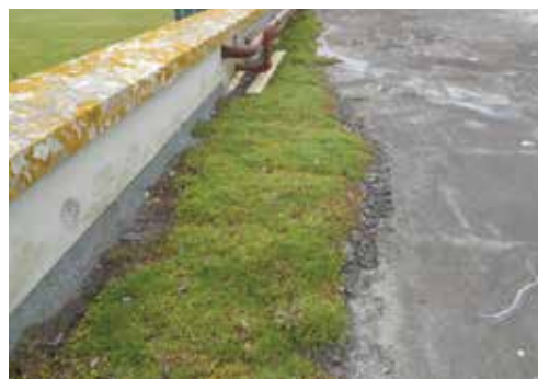
Top Temperature variations between ponded and dry areas can result in cracking.
