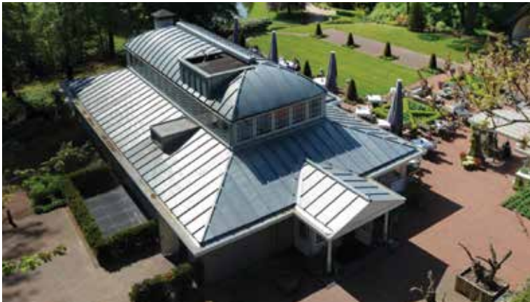
An example of natural zinc sheet roofing brings a crisp finish to roof detailing.
