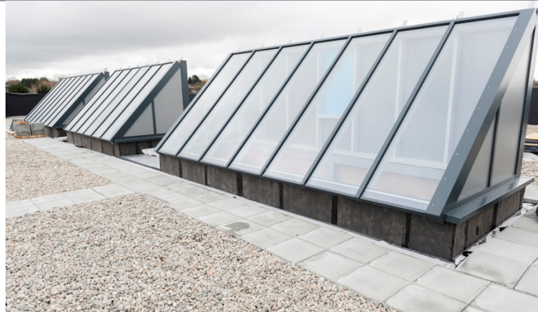
The roofing solution for all seven projects needed to overcome a number of specific design challenges
